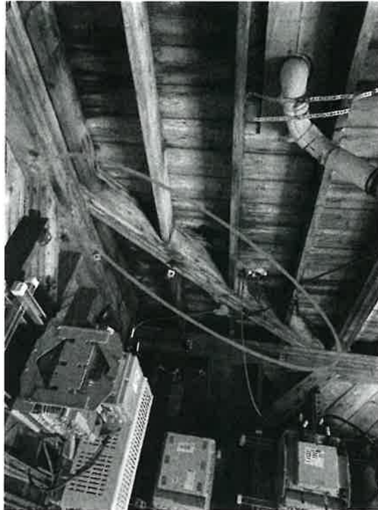
Photo 19: Belfry framing rotted bracing beams and poor joist end connections
