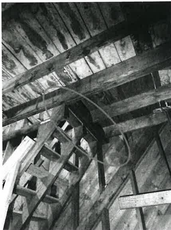
Photo 13: Notched joists and poor header connections
