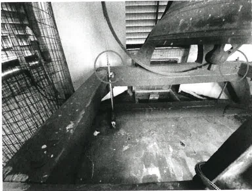
Photo 21: (2 of 4) Loose tension rods on the bell cradle
