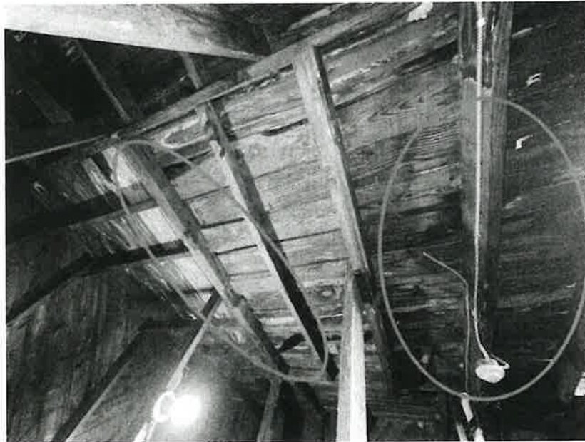
Photo 18: Water damaged floor planks and cut floor joist on level #2 floor framing
