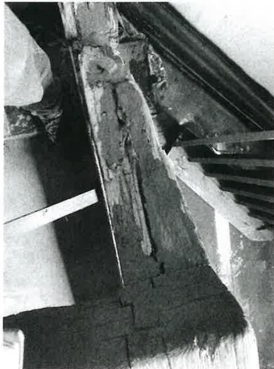
Photo 20: Rotted leg of the south end of the bell cradle
