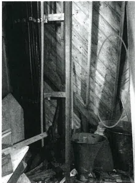
Photo 16: Slight water staining at level #1 west wall
