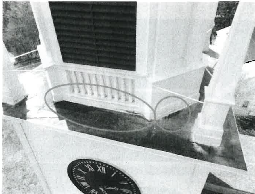
Photo 4: Standing water and detached sealant/flashing at east face belfry level
