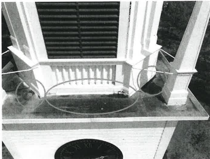
Photo 2: Standing water and deteriorating sealant at the west face belfry level
