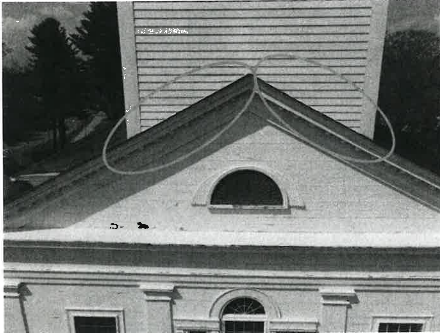
Photo 9: Suspect area with potential need for flashing (south face of tower)
