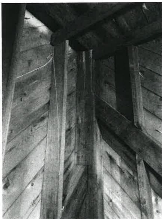
Photo 14: Toe nailed stud connections and minimal bracing connections
