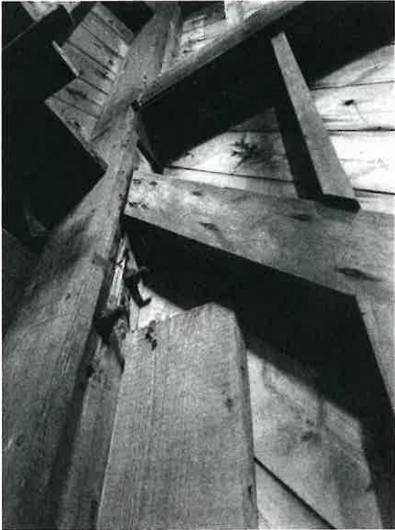
Photo 11: Splitting at the southeast post connection
