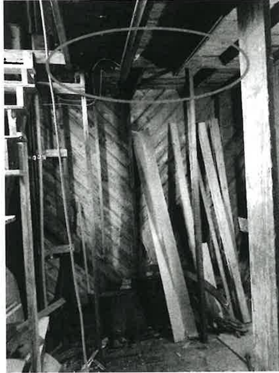
Photo 17: Poorly sized joists and beam members at level #2 floor framing
