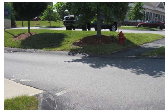
Poorly defined crosswalk
