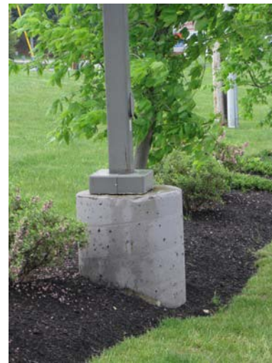
Incorrectly installed light post
