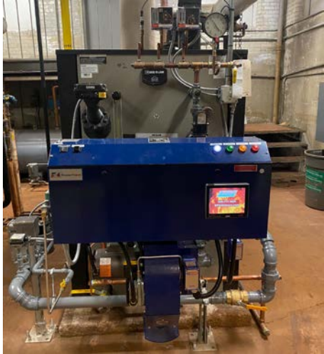
Town Hall Boiler
