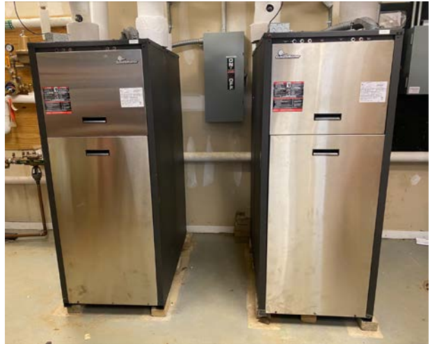
Senior Center Heat Pumps
