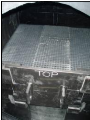
Figure 1. Removable bulkhead door across from ingress/egress ladder at rear of filtration chamber.
