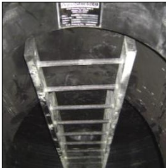
A permanent ingress/egress ladder provides access to filter chamber. Note metal product identification plate above ladder.
