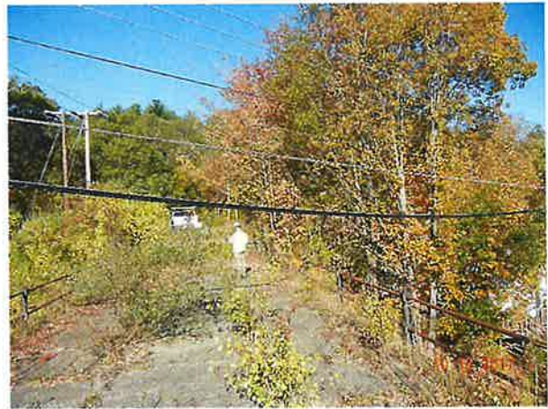
Photo 8: Low-Hanging Wires, Vegetation - West End of Bridge
