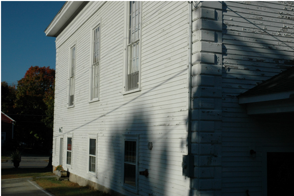
West Side Windows to have Replacement Shutters
