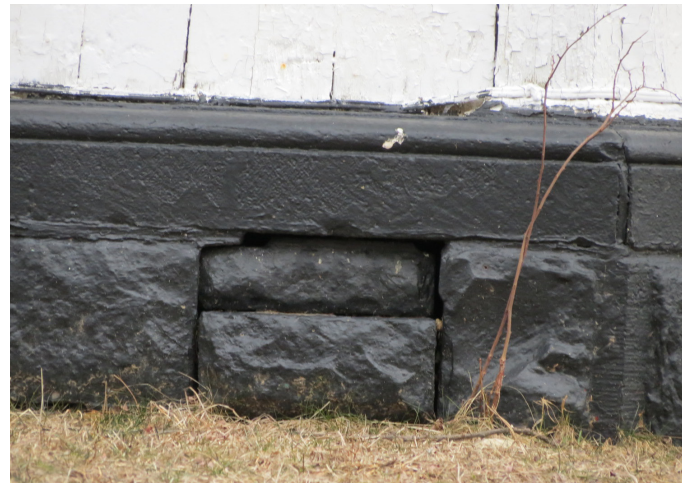
Figure 2.9: Displaced brownstone units at south foundation.
