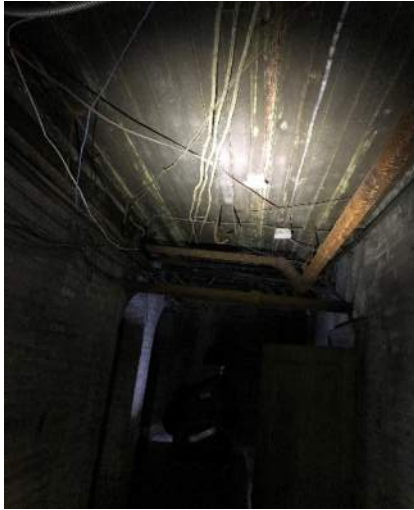
Existing wiring through corridor
