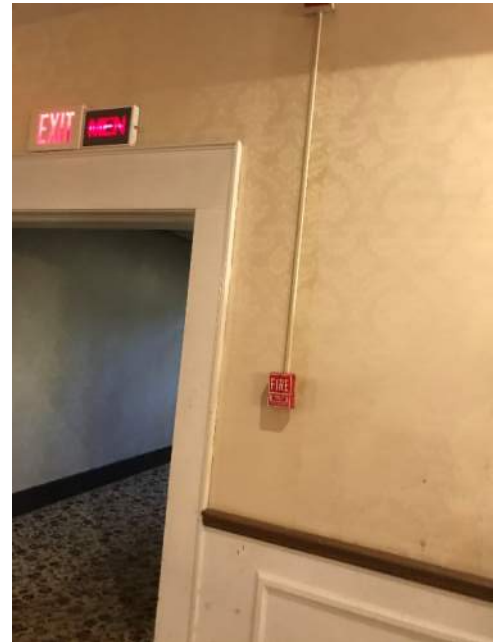
Exit sign, pull station and audio visual
