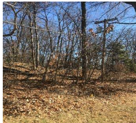
Pole mounted transformers
