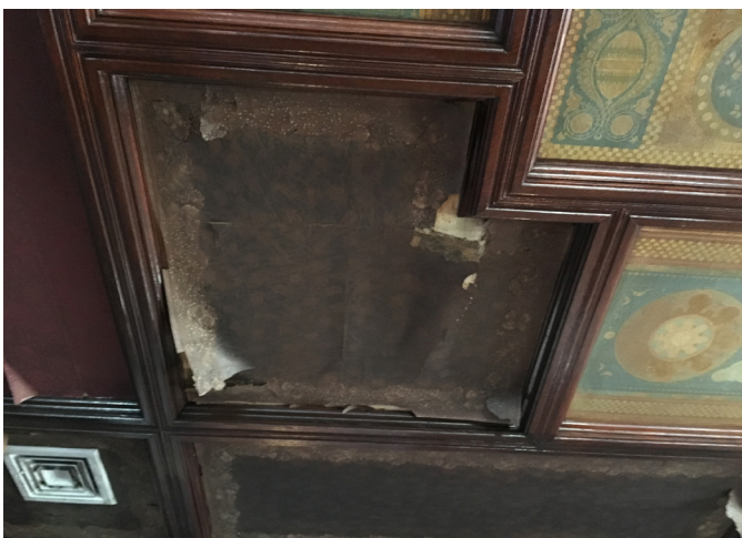
Figure 2.52: Failed replacement panel at second floor.
