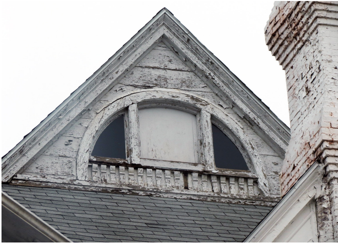
Figure 2.12: Typical deterioration at the upper gable of the south elevation.
