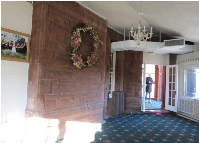
Figure 2.6: Exposed brownstone at the south elevation, inside porch.
