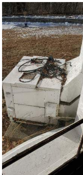
Existing Cooling Unit Serving the First Floor
