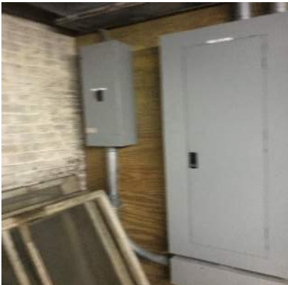
Panel B and Disconnect for Panel C
