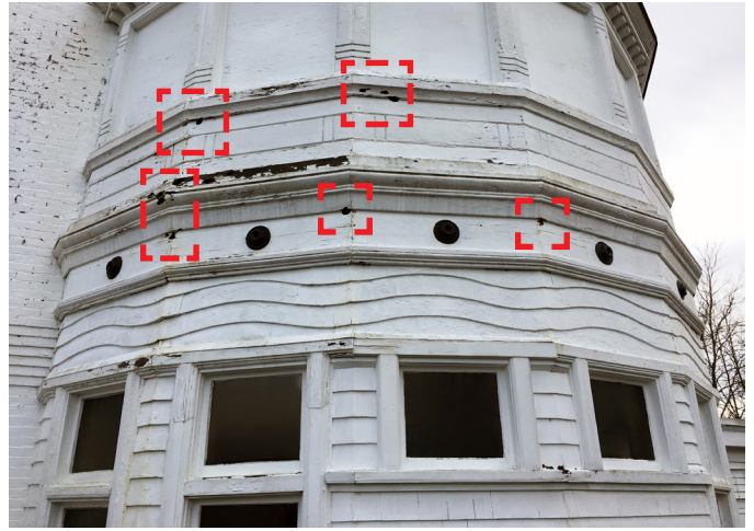
Figure 2.15: Woodpecker holes (indicated) at the northwest turret.
