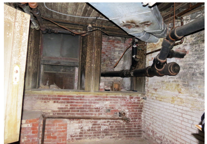
Figure 2.38: Interior view of areaway at the northeast corner, now enclosed by additions.
