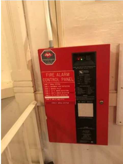
FACP located in the main lobby
