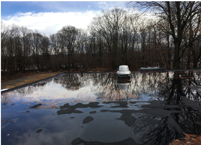
Figure 2.89: Ponding water at the roof of the ballroom addition.
