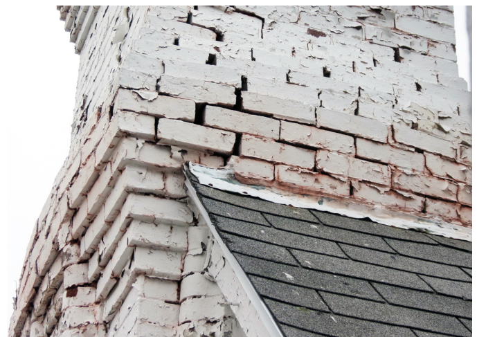
Figure 2.26: Displacement at south chimney
