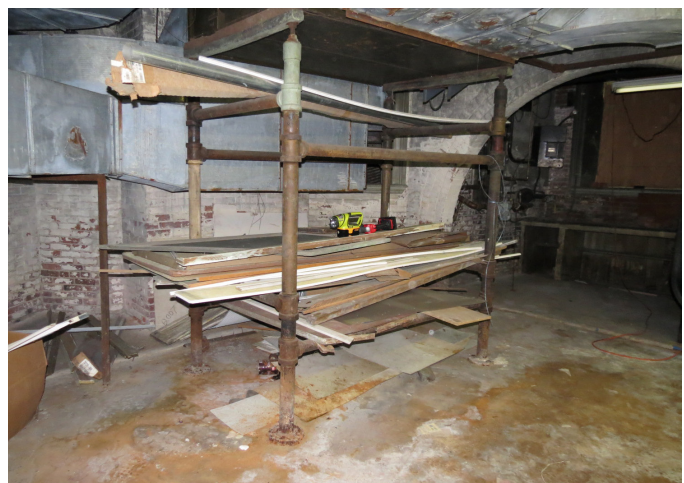
Figure 2.73: Evidence of water damage at basement slab.
