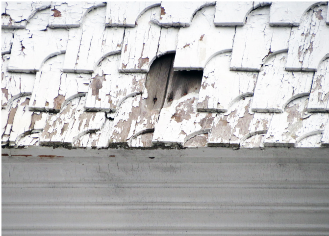
Figure 2.13: Severe deterioration at flared siding at the base of the second floor.
