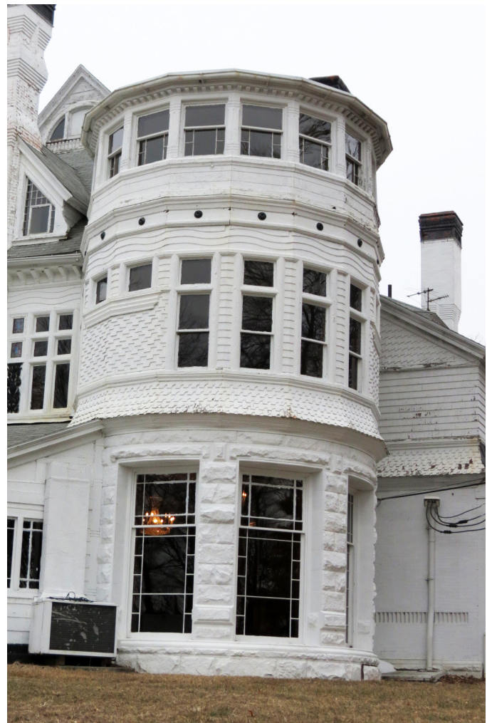
Figure 2.11: Southeast turret with four distinct shingle patterns exhibiting moderate deterioration.
