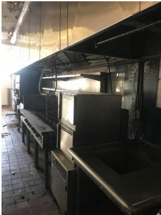
Ansul system in the Kitchen
