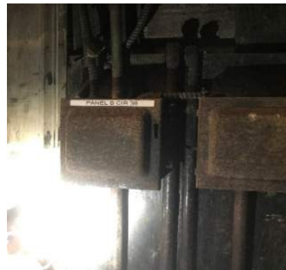
Disconnects for mechanical equipment
