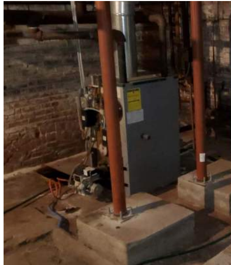
Primary Boiler Serving HVAC System
