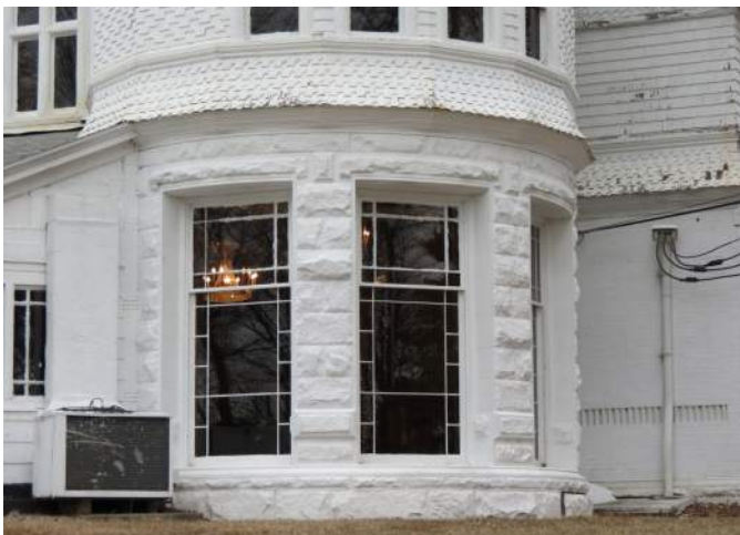
Figure 3.2: Vulnerable first floor windows at the southeast turret.
