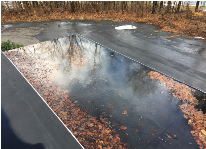
Figure 2.88: Ponding water at the roof of ballroom addition.
