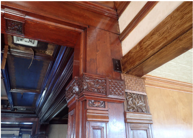
Figure 2.45: Mismatched woodwork at the second floor event space.
