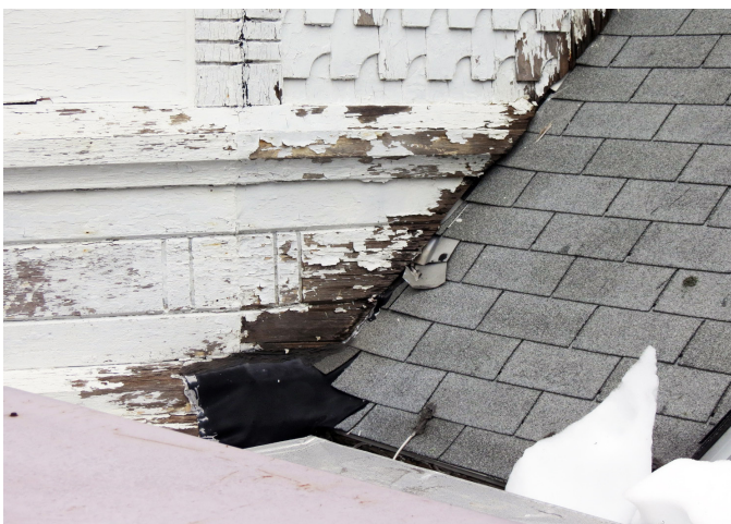
Figure 2.14: Severe deterioration at a siding-to-roof intersection.
