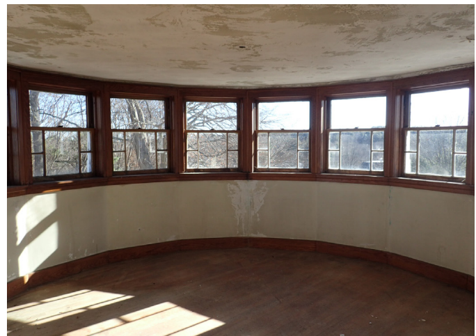
Figure 2.66: Third floor room at southeast turret, note plaster damage at ceiling.
