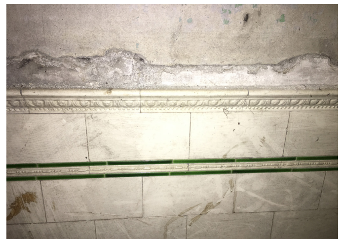
Figure 2.77: Tile at basement bathroom.
