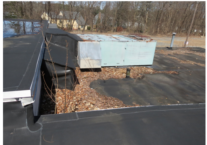
Figure 2.86: Area of active water infiltration at east addition roof.
