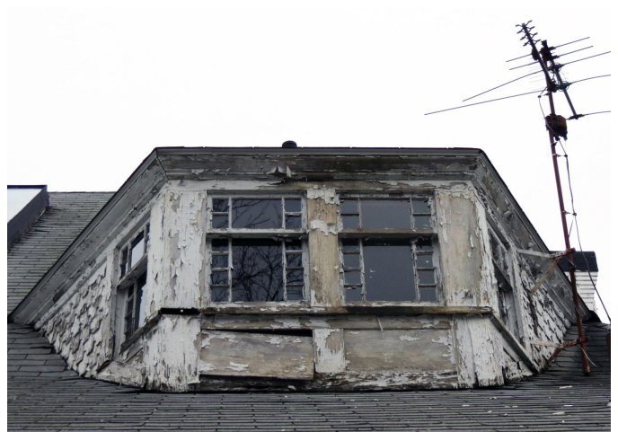
Figure 2.17: Severe deterioration of all wood components at the east dormer.
