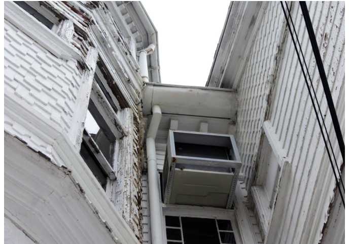
Figure 2.16: Severe deterioration adjacent to an undersized gutter.
