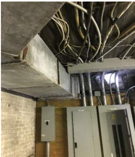
Wiring exiting the Panel A & Panel B
