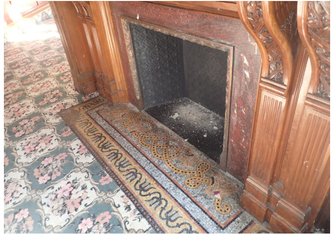
Figure 2.61: Detail view of mosaic hearth with minor damage in upper corner.
