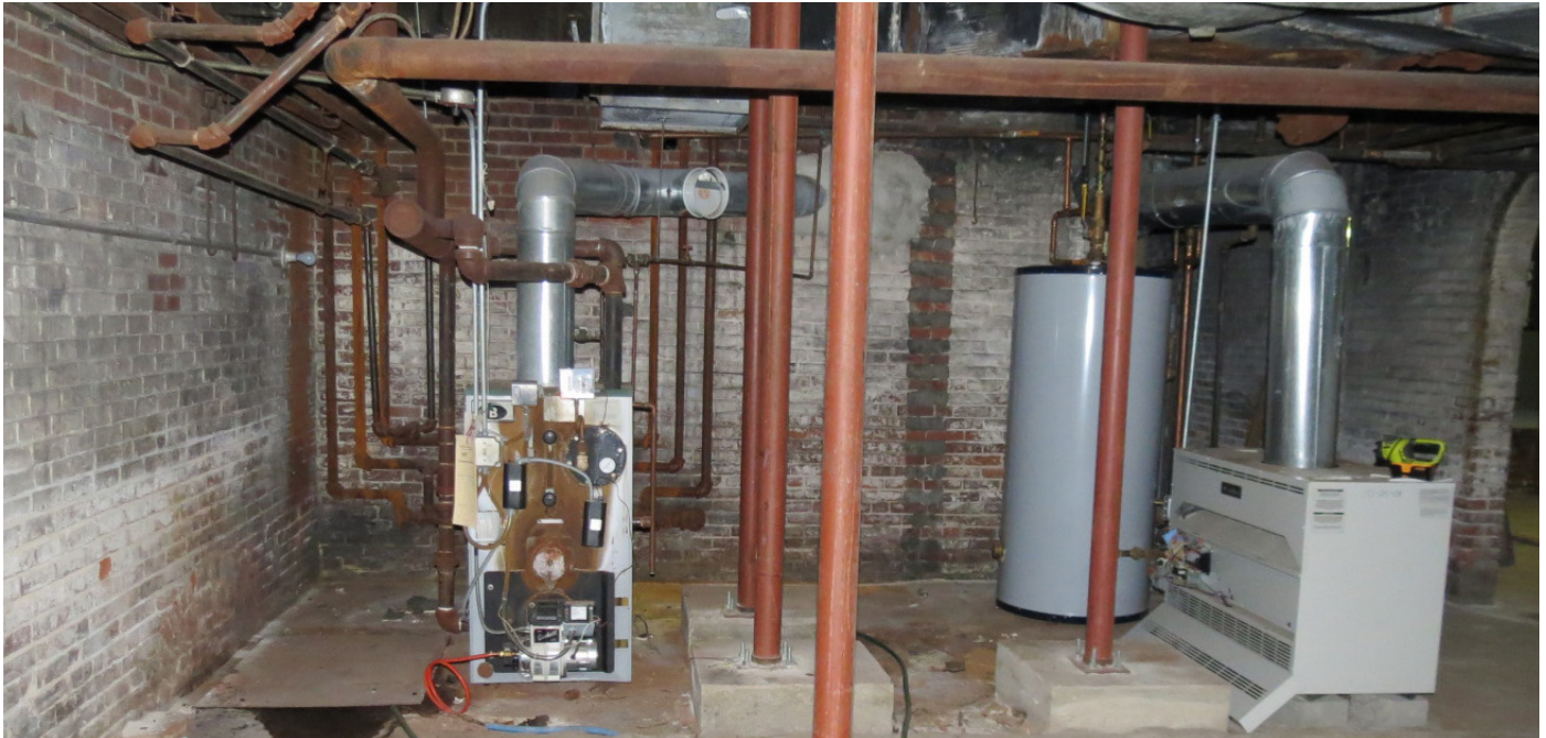
Figure 2.91: View of components of the existing mechanical and plumbing systems at the basement.
