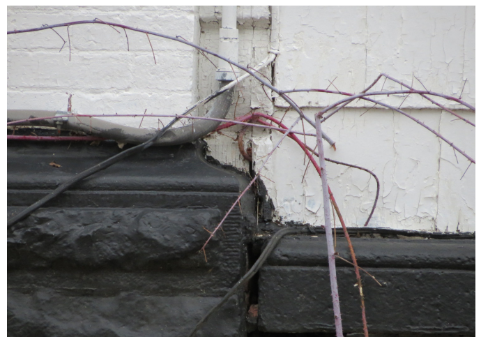
Figure 2.10: Open joint between brownstone foundation and porch construction.
