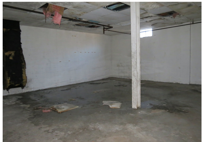
Figure 2.87: Result of active water infiltration at east addition roof.
