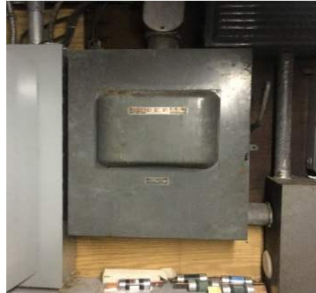
Main Service Disconnect
