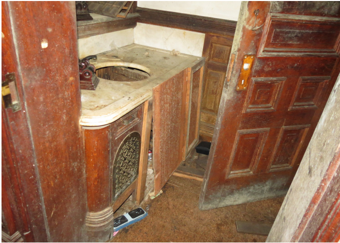
Figure 2.44: Deteriorated woodwork at the first floor bathroom.
