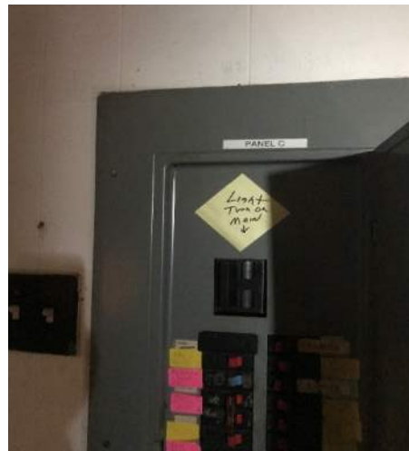
Panel C located in the main Kitchen
